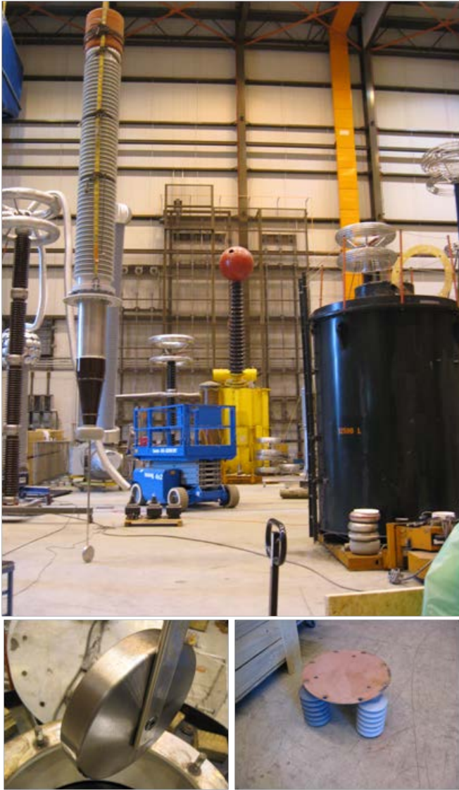
Figure 1. Bushing shield (22 cm dia.) stainless steel electrode attached to 1800 kV BIL bushing. Ground plate electrode is connected to and raised off the tank bottom.
