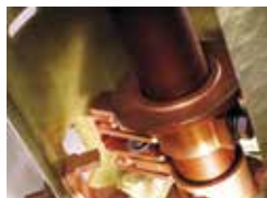
LRT-200-2 Selector Switch
