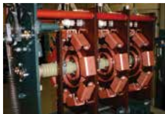
GE LRT-68 Load Tap Changer
