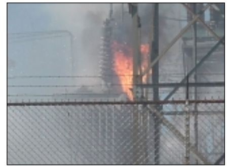
Significant transformer fires have been reported despite established safeguards
