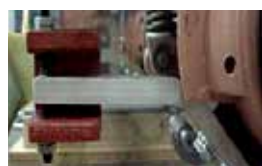
Transfer Switch Stop Adjustment
