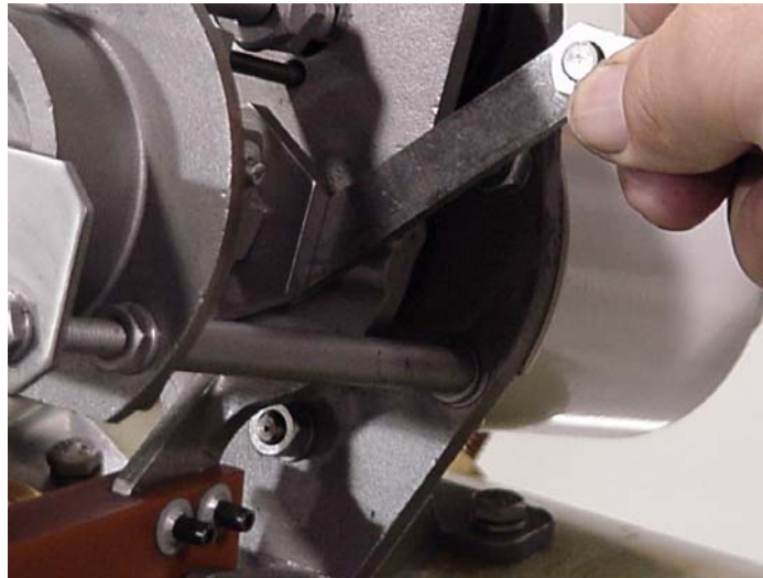
Fig. 1: Checking the interrupter bottle pre-travel
