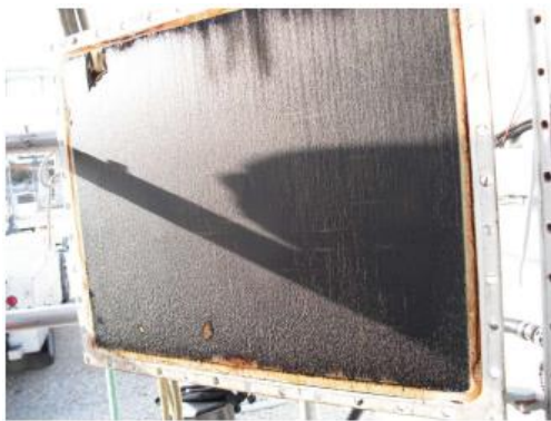
Sludge On Inside of Door
